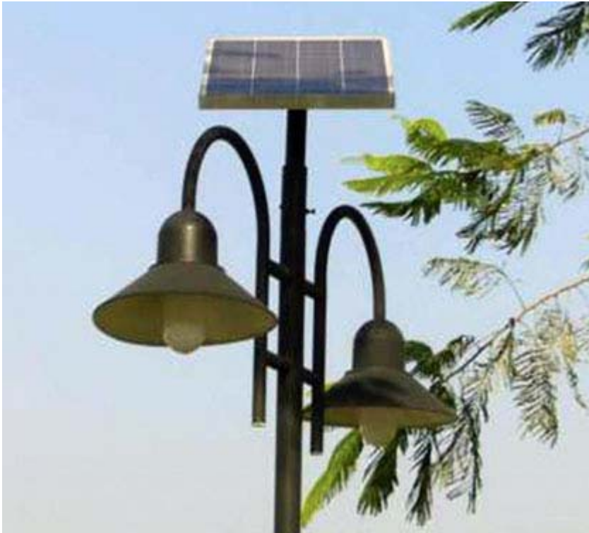
■ Solar Panels Installed for External Lighting
