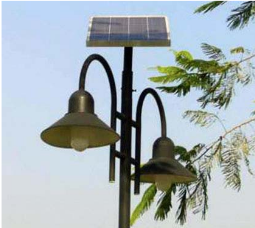
■ Solar Panels Installed for External Lighting
