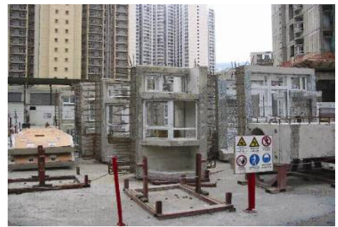
Precast Element Storage Yard
