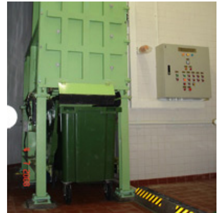
Small Scale 'Distributed Compactor System' installed in each domestic building
