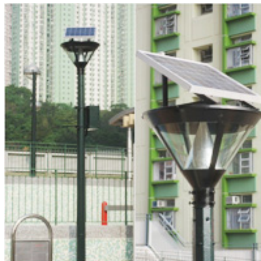
PV Pole Lamp
