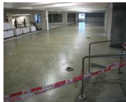
Tin Heng Car Park - Renovation on the first, second and fifth floors to a Telebet cum Volunteers and Training Centre
