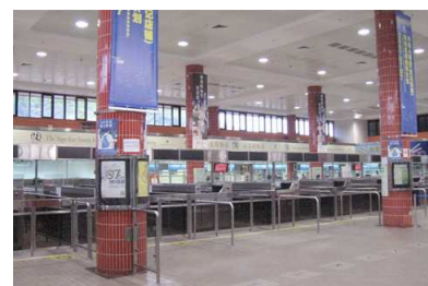
High energy efficiency fluorescent lamps were installed at new arrival hall at Lo Wu Control Point.
