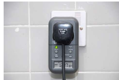
A seven-day timer switch installed for electric appliance in office common area.
