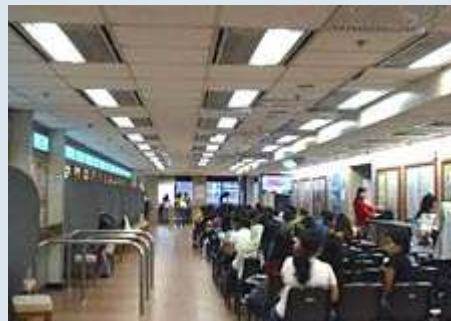
The illumination level at public waiting area was adjusted to about 300 lux as recommended by EMSD.
