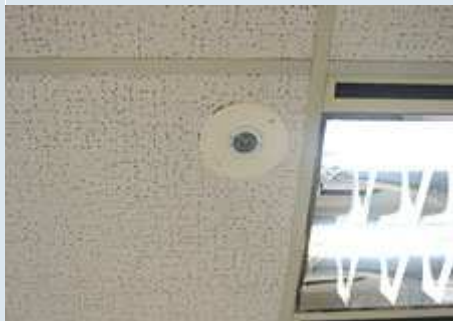
Occupancy sensors were installed at 17 cellular offices at the Immigration Headquarters.
