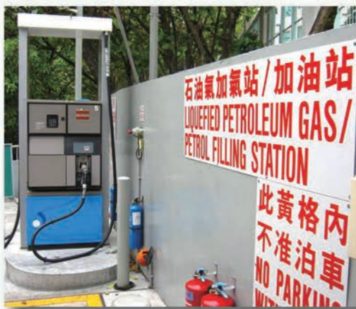
▲ A Petrol Filling Station with LPG filling facilities
