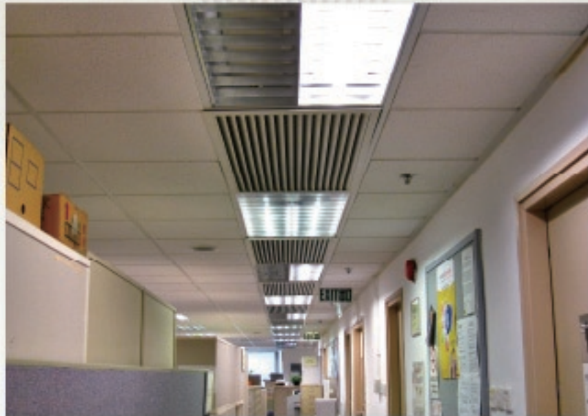
Illumination level in common area can be adjusted down by removing excessive bulbs or fluorescent tubes
