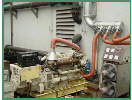
Exhaust Gas Extraction System in the Engine Testing Yard
