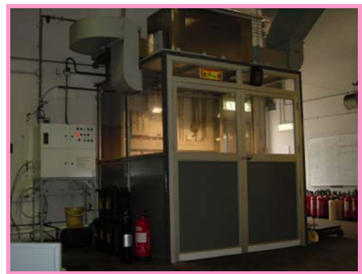
Odour Treatment and Air Disinfection System fitted in the Fire Extinguisher Workshop
