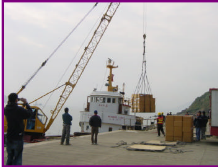
Monitoring the discharge of Class 1 Dangerous Goods (Fireworks) at Hong Kong Disneyland Service Pier
