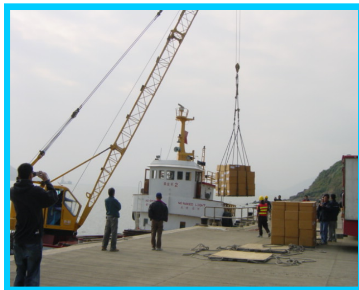
Monitoring the unloading of Class 1 Dangerous Goods (Fireworks) at Hong Kong Disneyland Service Pier
