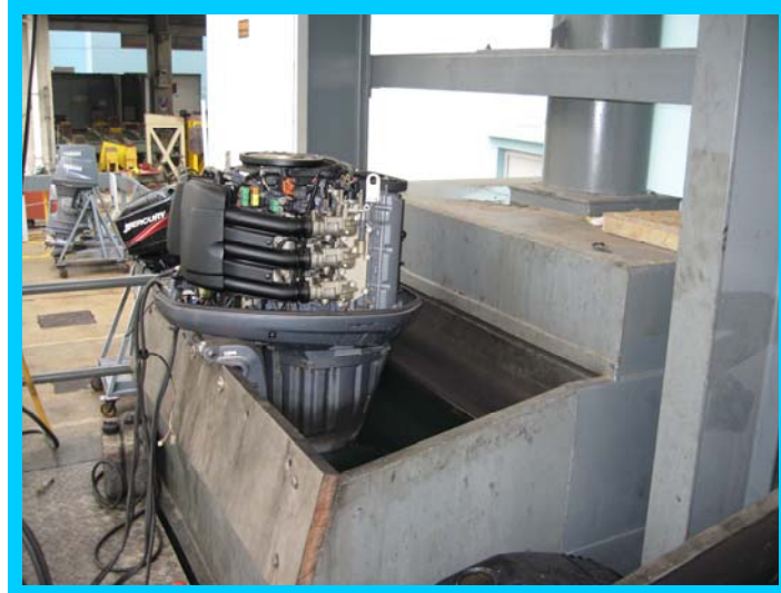
Exhaust Gas Extraction System to Remove Exhaust Gases Emitted during Engine Testing Operations
