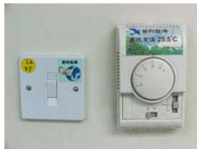
Energy-saving labels on switches
