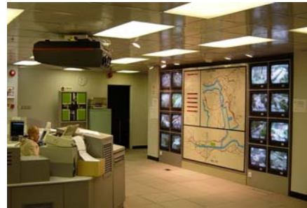
ATC Control Room
