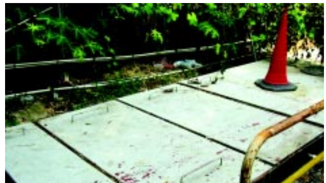
工地化糞池 Septic tank at site office
