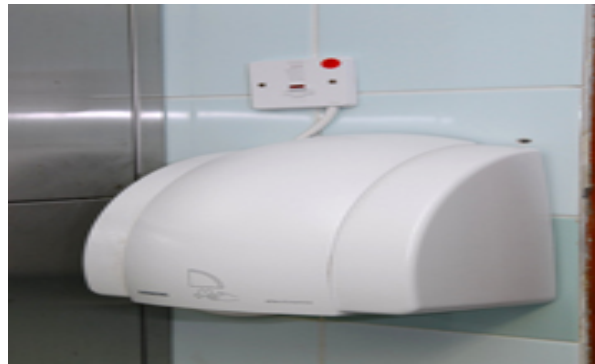
Hand-dryers are installed in toilets to encourage less use of tissue paper.
