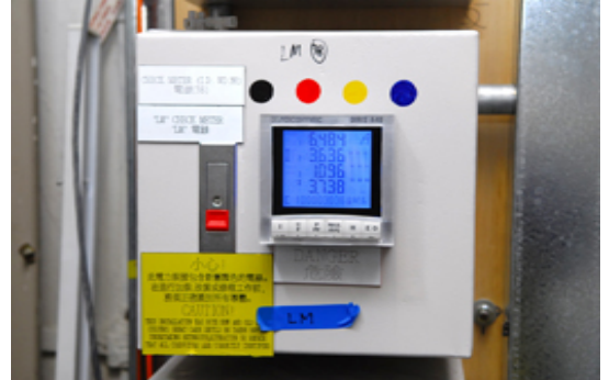
Meters are installed to monitor the electricity consumption of the floor.
