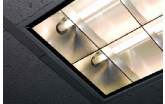
Thin fluorescent light tubes (T5) are used to reduce power consumption.
