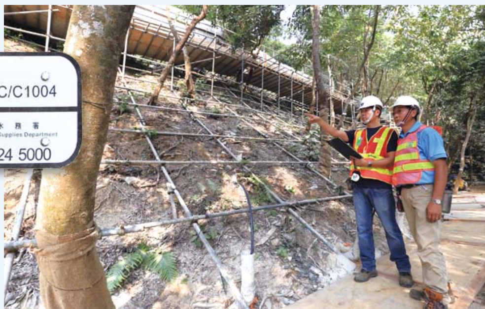
現場監督位於沙田筆架山的斜坡鞏固工程 Site supervision of the slope upgrading works at Beacon Hill, Shatin
