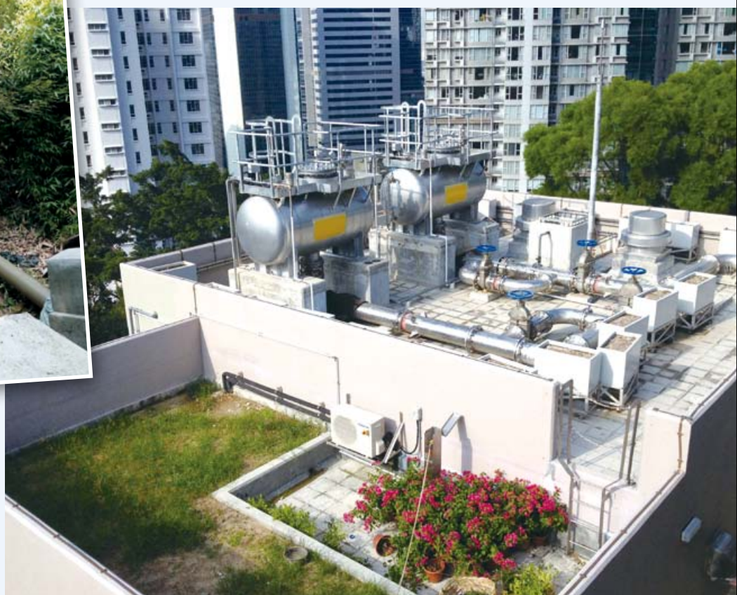
寶雲徑海水抽水站 Bowen Drive Salt Water Pumping Station
