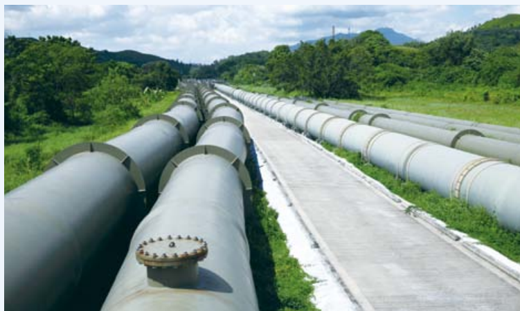
大型水管輸送東江原水 Huge pipelines conveying Dongjiang Water
