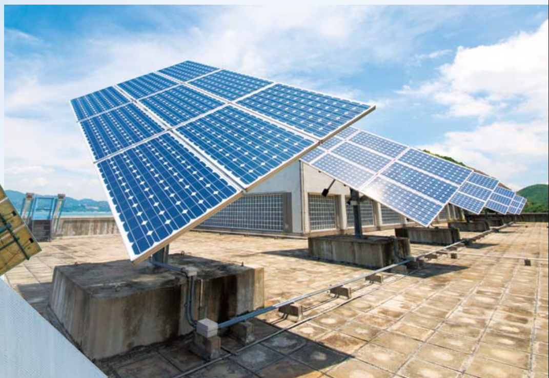
位於欣澳海水抽水站的太陽能板和風力發電裝置 Solar panels and a wind turbine at Sunny Bay Salt Water Pumping Station
