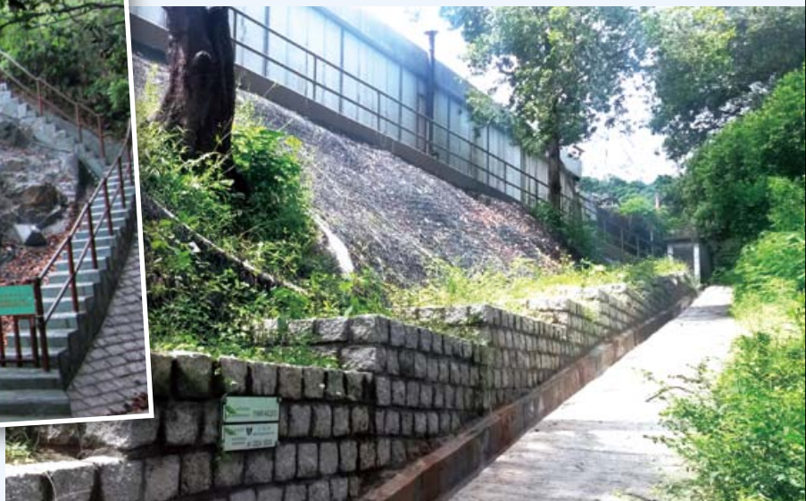
位於葵涌九華徑的斜坡已完成斜坡鞏固工程約一年 Upgrading works of the slope at Kau Wah Keng, Kwai Chung has been completed almost a year
