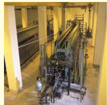
將濾出的廢物製成泥餅的壓濾機。 Filter press for converting treatment waste into sludge cakes.
