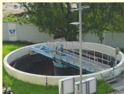
濾水廠內的污泥濃縮池，經濃縮後的污泥會被送往壓濾機進行最後脫水程序。 Sludge thickening tank in water treatment works for thickening the sludge before final dewatering by filter press.
