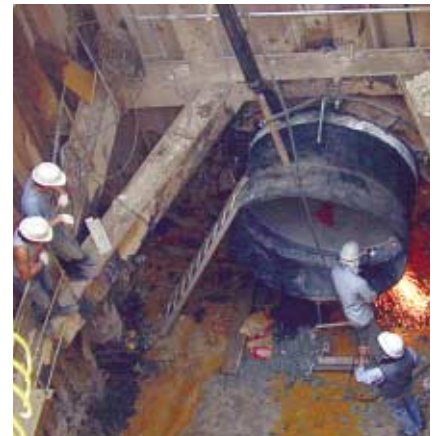
採用無開掘式方法安裝水管。 Installing new pipes with trenchless method.
