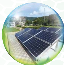
廈村污水泵房的太陽能光伏板 PV panels at Ha Tsuen Sewage Pumping Station
