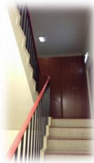
Figure 6: Lighting with motion sensors
