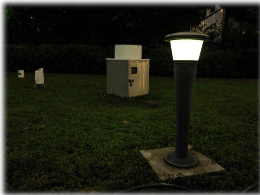
Figure 8: Solar energy lighting device
