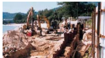
沿東灣頭路的污水渠敷設工程 Construction of sewer along Tung Wan Tau Road
