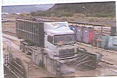
在工地出口處設有車輪清洗站，以確保車身不會帶出泥塵。 Wheel-washing facilities at site exits to remove any sticky material from vehicles.
