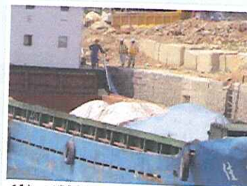
在運載物料上貨車蓋上帆布 Covering the material by tarpaulin on barge during delivery
