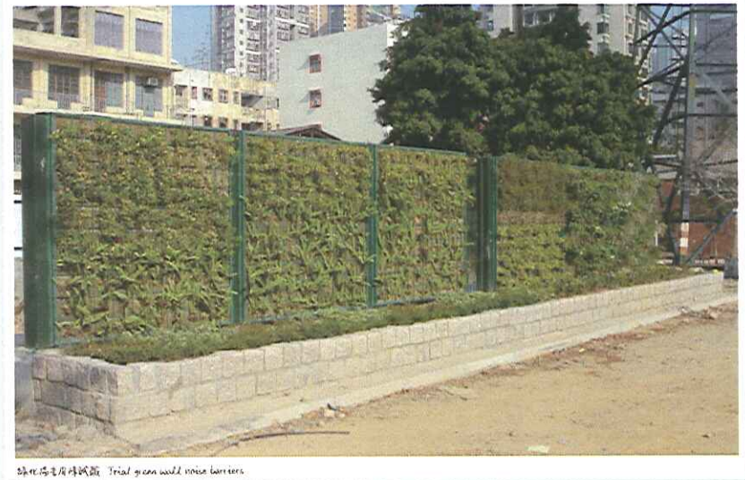
綠化牆噪音屏障試驗 Trial green wall noise barriers
