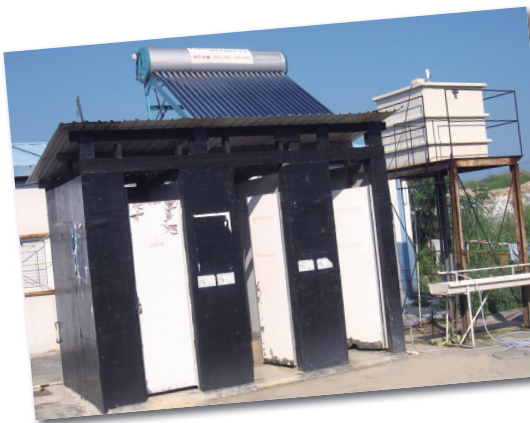
工地內設置的太陽能熱水系統 Solar powered water heating system on works site
