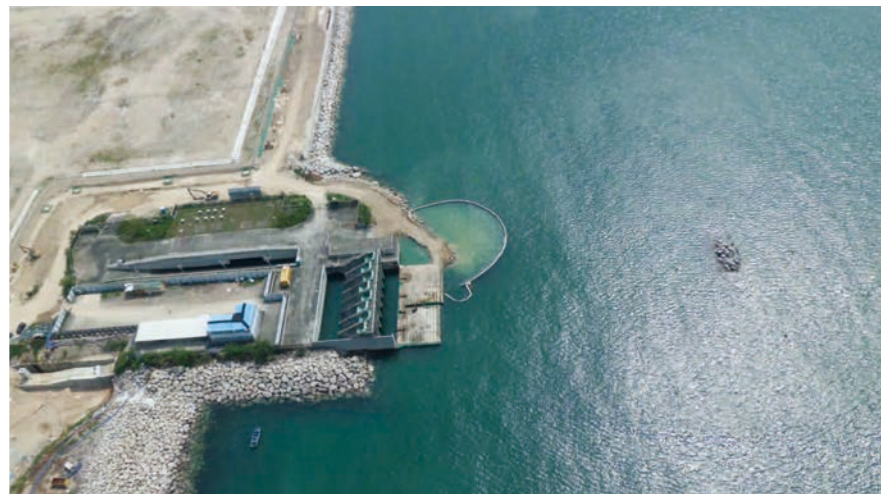
將軍澳市中心南及調景嶺的基礎設施 Infrastructure Works at Tseung Kwan O Town Centre South and Tiu Keng Leng 使用隔泥幕緩解海事工程對水質的影響 Use of silt curtain to mitigate impacts on water quality during marine works
