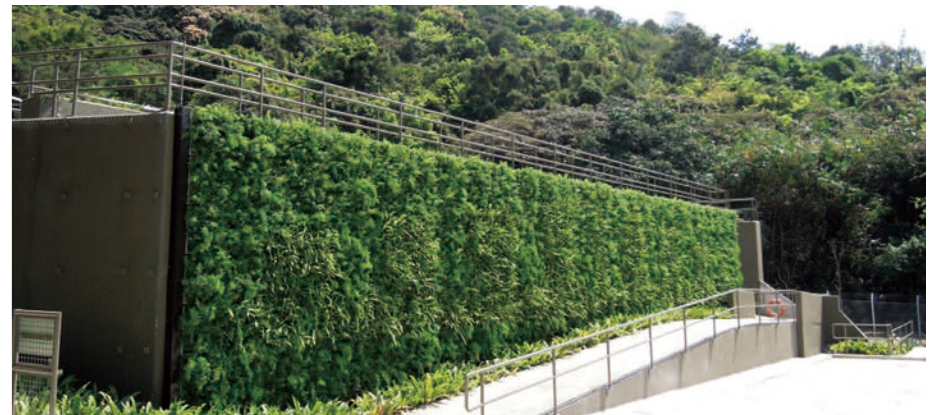
斜坡工程 Slope Engineering Works 泥石壩的可持續垂直綠化牆 Sustainable vertical green wall of check dam
