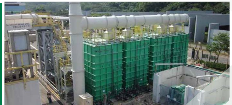
◆ 生物滴濾塔 Biotrickling Filter
