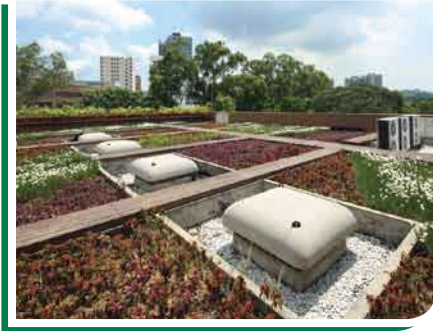
● 舊墟污水泵房的綠化天台 Green roof at Kau Hui Sewage Pumping Station Compound
