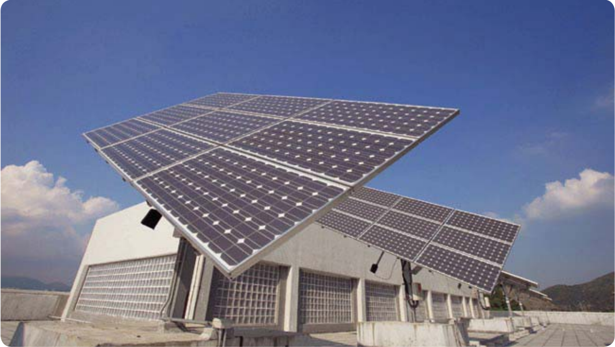
設於欣澳海水抽水站的再生能源系統。 A renewable energy system is in use at Sunny Bay Salt Water Pumping Station.
