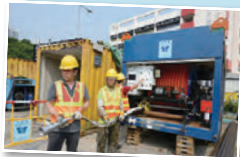
水管修復－內層噴霧塗搽技術 Pipe rehabilitation work – spray applied lining
