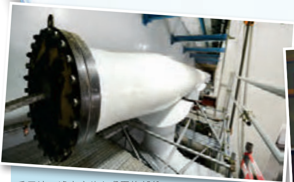
重置沙田濾水廠的主喉更換部份 Replacement of delivery mains under reprovisioning of Sha Tin Water Treatment Works
