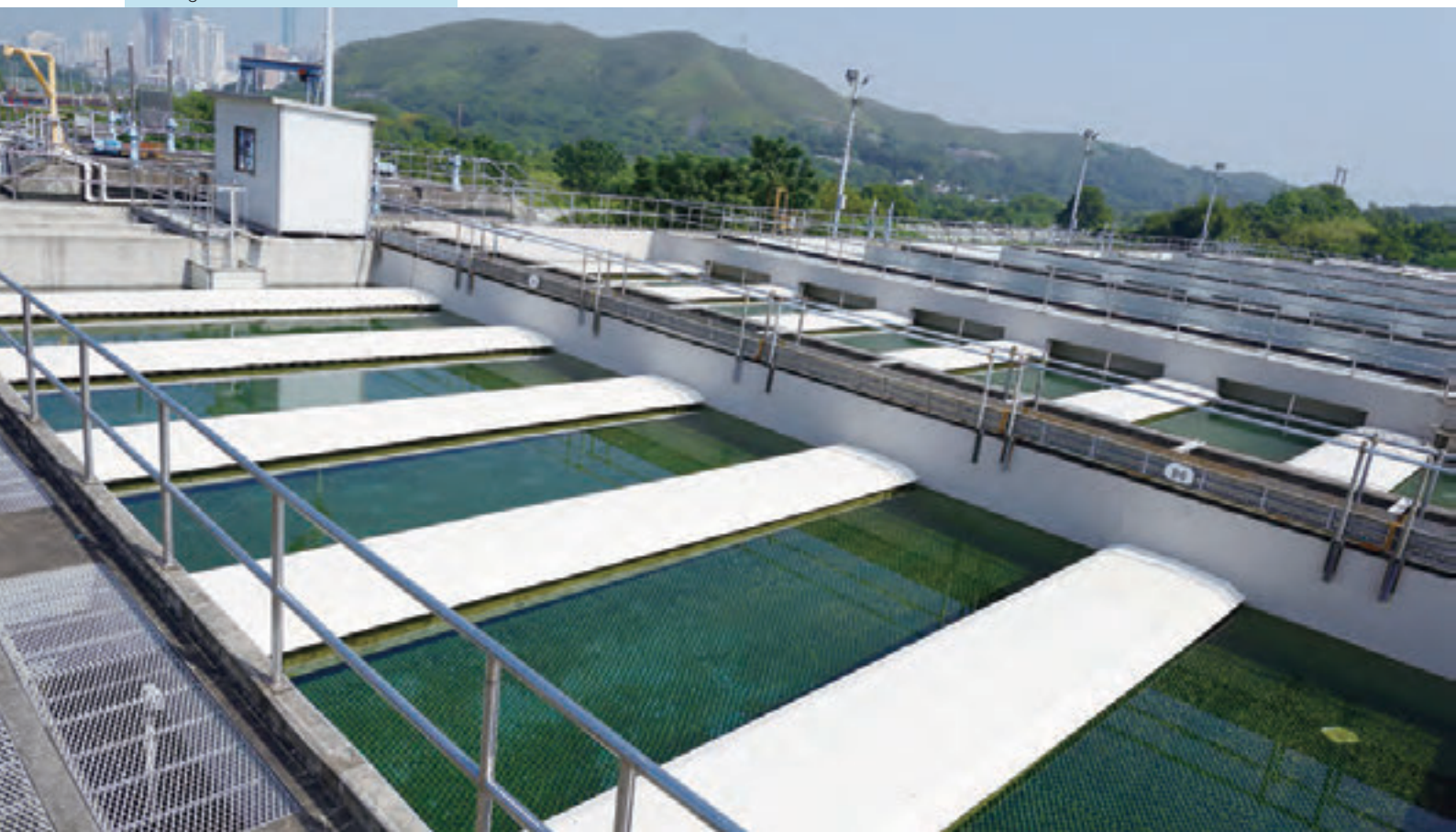
上水濾水廠澄清池內的斜管 Inclined tubes at clarifier of Sheung Shui Water Treatment Works
