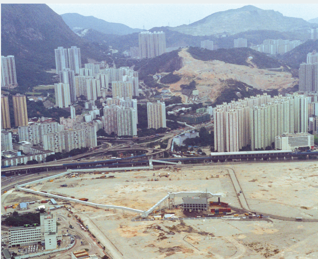
彩雲道及佐敦谷的地盤平整工程 - 輸送帶系統 Site Formation Project at Choi Wan Road and Jordan Valley - Conveyor Belt System
