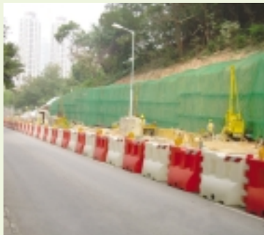
在土坡架設防塵網 Protective netting for suppressing dust emission at soil slope
