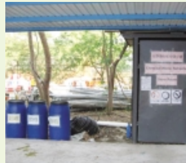
化學廢物臨時貯存設施 Chemical Waste Temporary Storage Facilities
