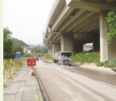
定期清洗工地旁的公用道路 Regular cleaning at public road adjacent to the work site
