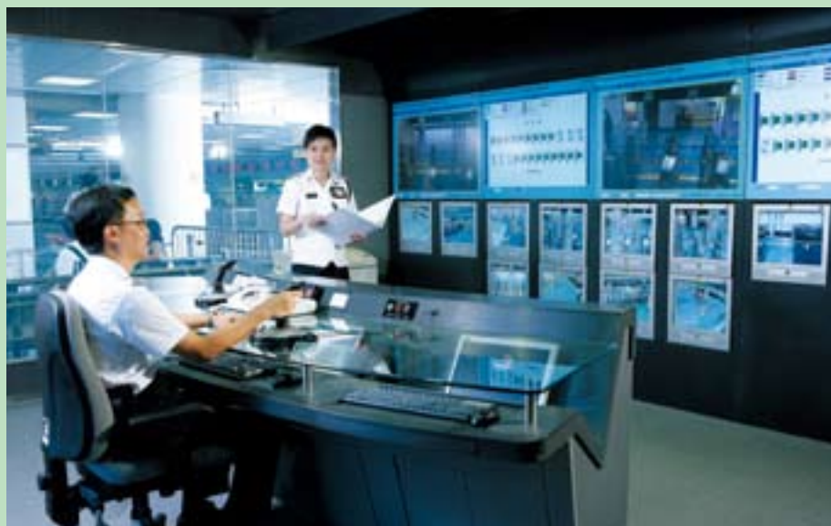
港澳客輪碼頭管制站的e-道控制室。 The e-Channel control room at the Macau Terminal Control Point.
