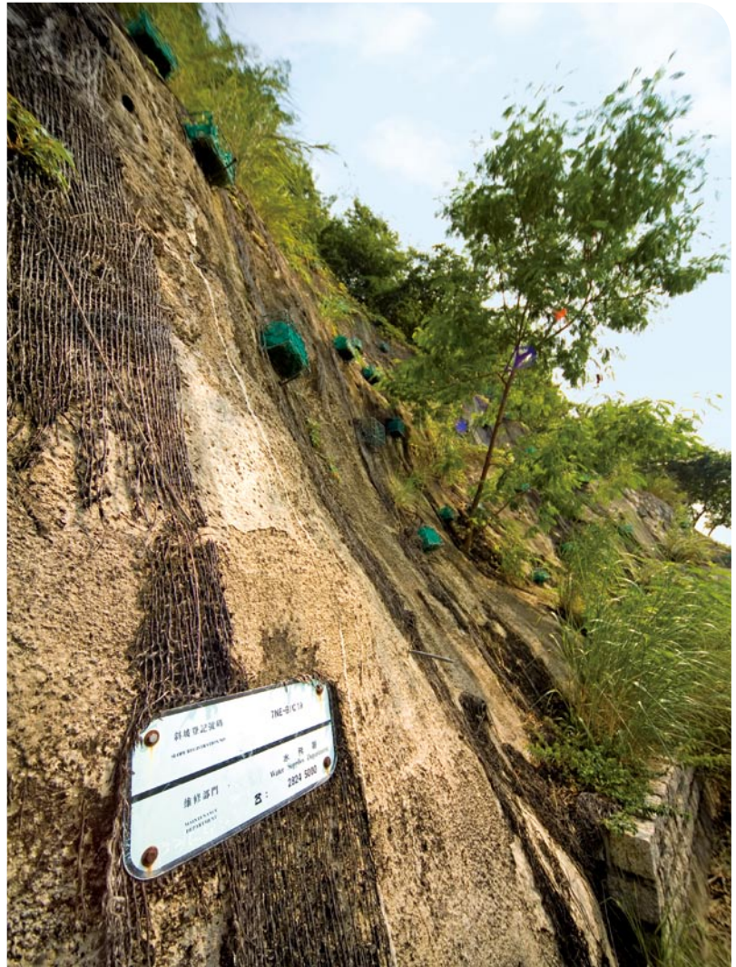
水務署負責維修的6000多個斜坡中其中一個。 One of the over 6000 slopes for which WSD is responsible.
